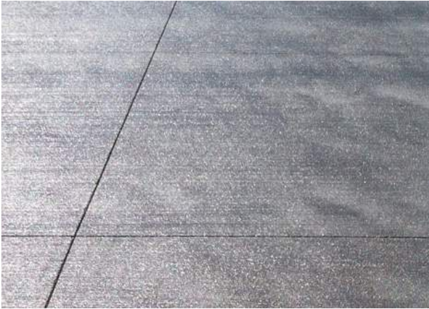
Surface type A - Brushed Concrete - U5/U6 Deep textured wire broom finish - 5% black oxide - decorative saw cuts to be included and specified in detailed design.
