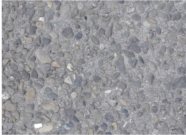
Surface type B - Exposed aggregate concrete - 16mm awatoto with awarua pebble 5% black oxide - decorative saw cuts tbc in detailed design.
